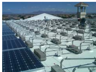
GCS K8 Solar Project
